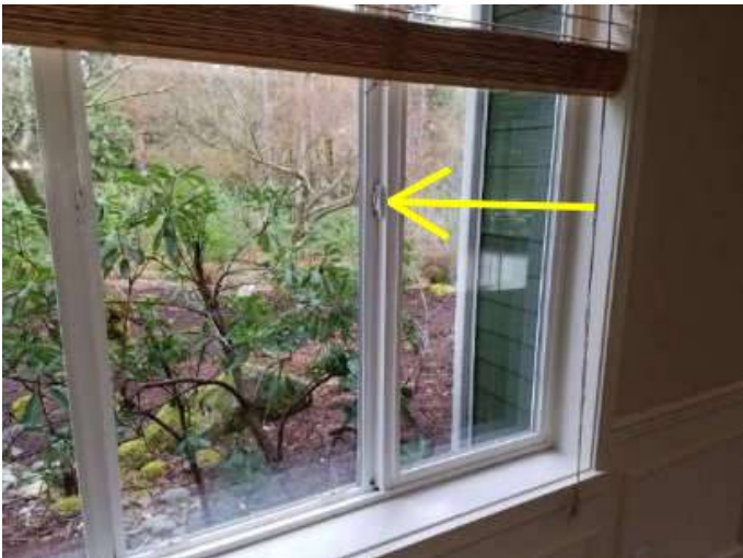
Photo 26-1 Loose lock mechanism in the living room
