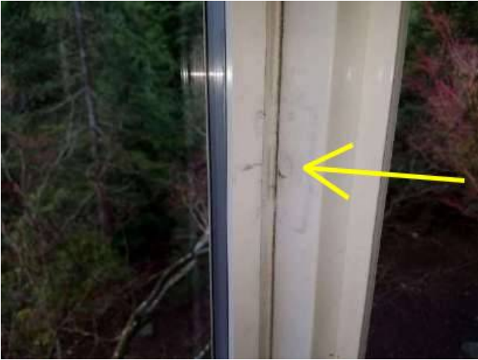
Photo 26-2 Lock mechanism missing in the 2nd floor NW bedroom
