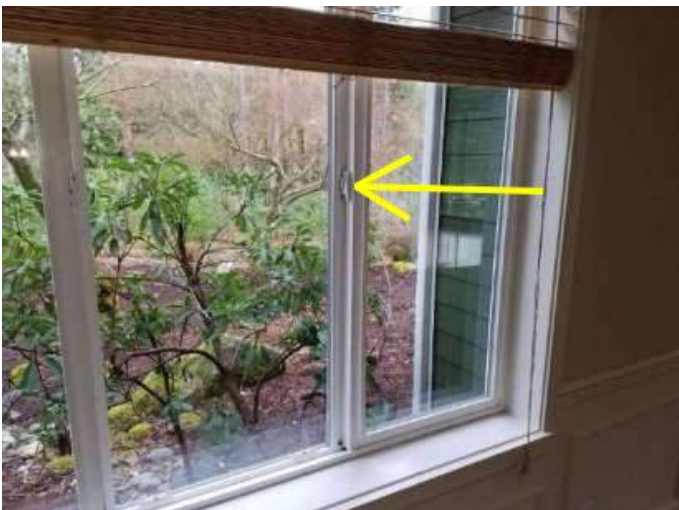
Photo 26-1 Loose lock mechanism in the living room
