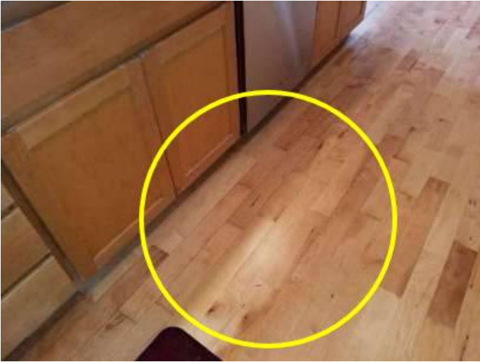
Photo 28-1 Kitchen floor in front of the sink and dishwasher
